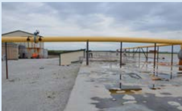
Includes a 7.5 million-gallon digester
