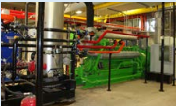
Generates 1.06 MW of electricity
