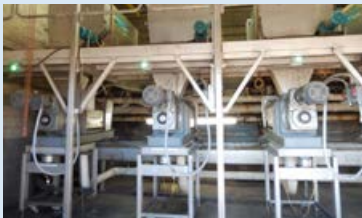
Processes digester effluent
