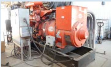
Generates 1.42 MW of electricity
