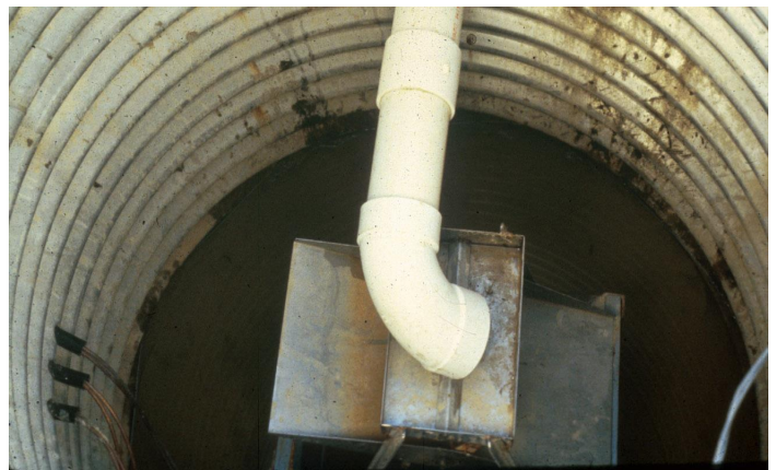
Photo 2. Tipping bucket flow gauge, to measure drainflow
