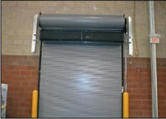
Air curtains prevent flying insects from entering the processing building through receiving, shipping, or employee entrances. Photos courtesy of Mars Air Doors (Gardena, Calif.).
