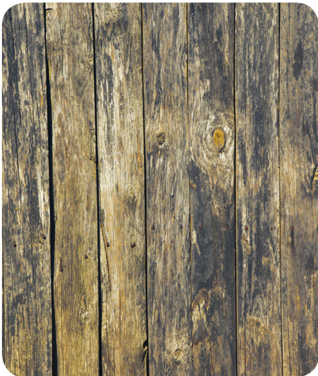
Figure 1. Porous wood, corroded metal, flaking paint, and carpet are materials that should not contact fresh produce. These materials are rough or absorbent, so they can't be easily cleaned or sanitized. Use smooth plastic, metal, or painted materials instead.
