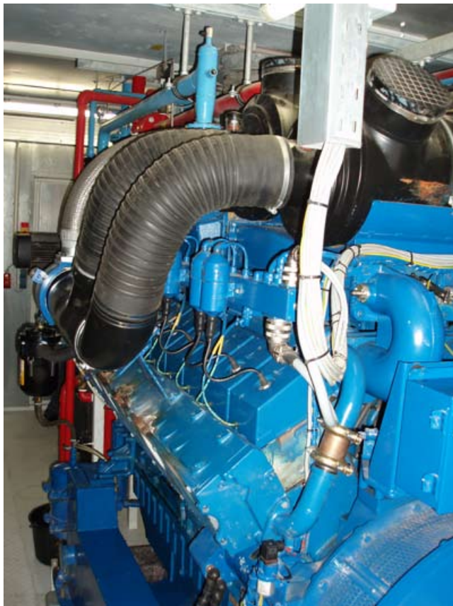
Electric generation unit showing piping for recovering heat that is used to heat up the AD reactor.
