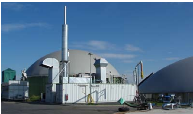
Two anaerobic reactors (foreground) showing flexible covers to collect gas as part of a community AD system in Juehnde in Southern Lower Saxony, Germany. Also shown: housing for an electric generation set and an underground mixing tank.
