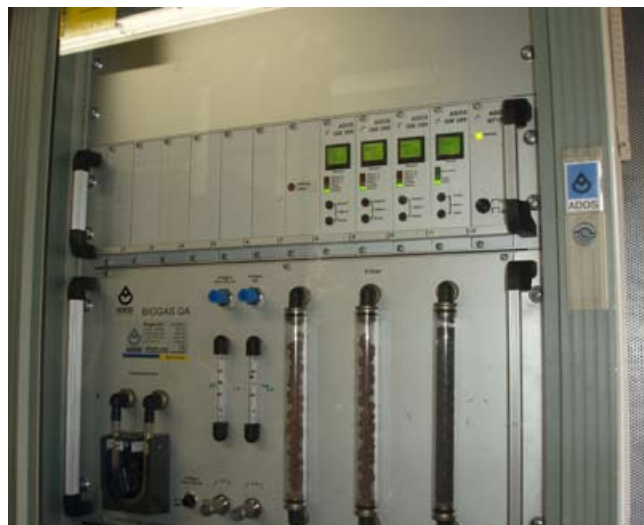
Control panel for biogas monitoring.
