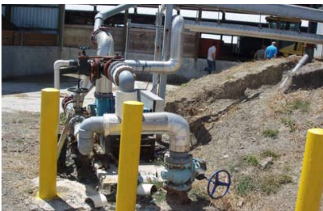
Piping for transporting digested liquid manure effluent from the AD reactor to an open lagoon on a farm in Oregon.
