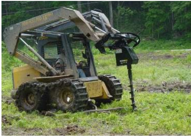
Figure 11. The versatile skid steer, mounted with an auger, can be used to plant trees on rougher terrain, in rockier soils, and around logging slash and stumps where machine planters would not work.
